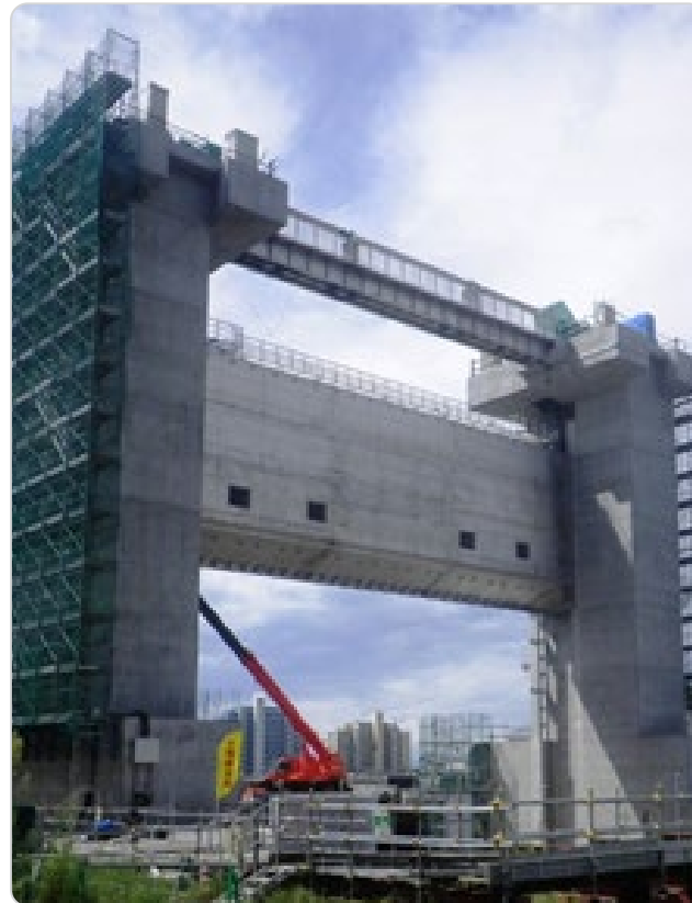
Flood gate. Picture courtesy of NSSC.
